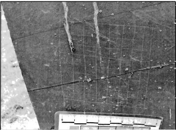
Although slate is hard, it is not immune from graffiti. Here a vandal has inscribed a checkerboard on the back of a stone.
