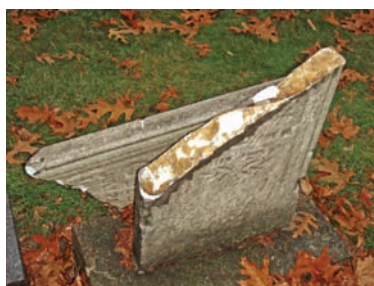
A typical “simple” epoxy repair that was doomed to failure. This inappropriate repair will make a correct repair more time consuming — and costly.
