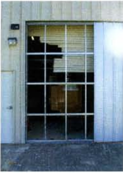
Roller doors frequently failed as a result of wind-induced damage and poor design (photo credit: Christopher Letchford, Texas Tech)
