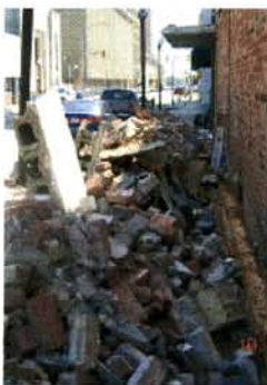
Brick veneer failure due to wind forces.
