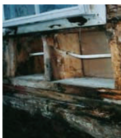
The consequences of inadequate moisture control in a historic structure can be severe.
