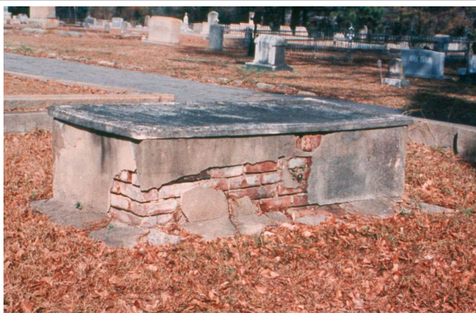
Example of modern concrete stucco coming off in large sheets.
